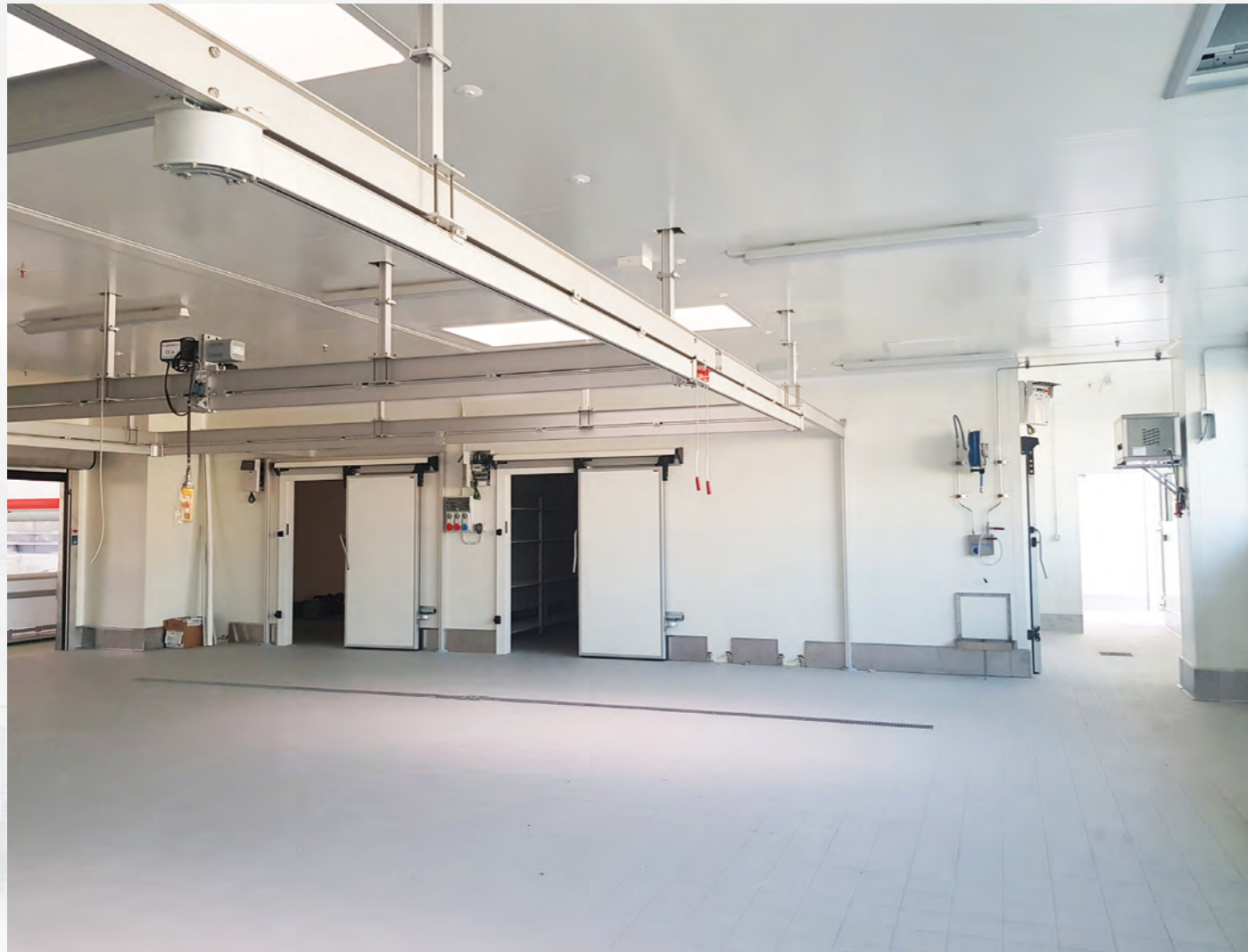
Celle con guidovia \ Cold rooms with rail passage
